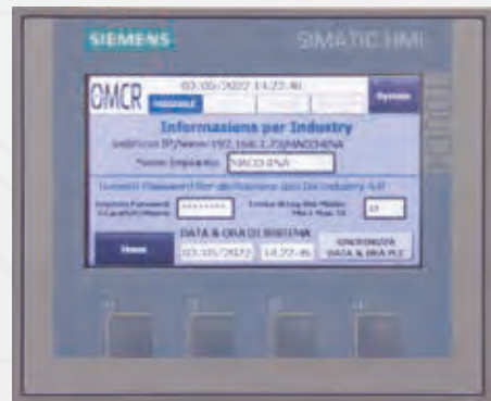
Control panel - detail
